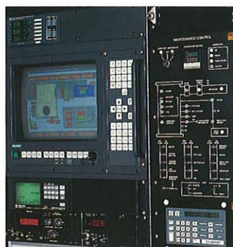
SSC-600 System controls
